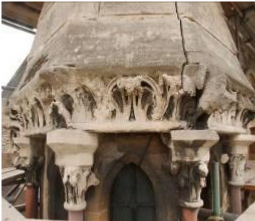
The north west stair turret; structural movement and severe weathering of stonework is the result of poor weather detailing to the stone roof of the stair turret. The deterioration of the supporting capitals has contributed to the movement of the roof.
