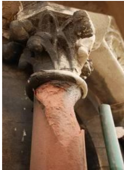
An example of the severe deterioration of the stonework at the church.
