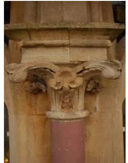
Works in progress: the repair and consolidation of a capital to the west gable of the nave.
