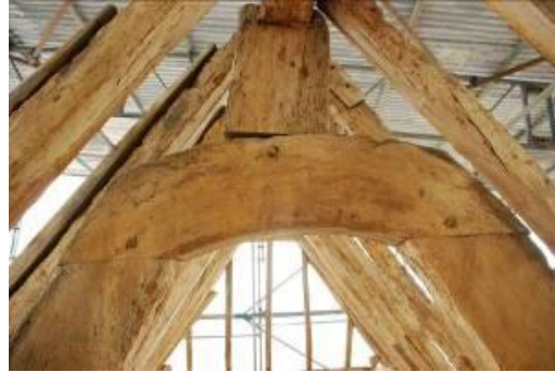
Detail of the apex to one of the cruck cross frames, showing oak timbers over 600 years old in excellent condition
