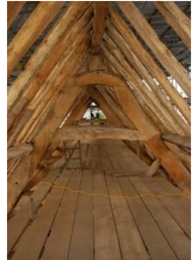
View of the barn in the process of repair that will prolong the life of this outstanding building.
