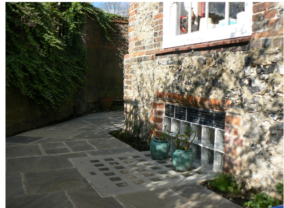
The new pavement light and glass block window that have transformed the cellar.
